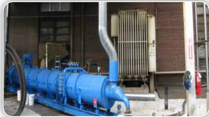
Full-scale prototype sorbent activation unit, installed at a power plant.
