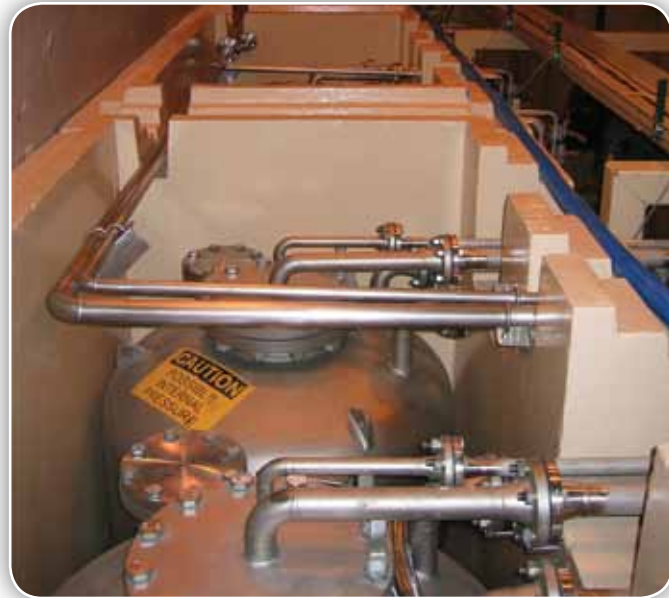
Liquid radwaste processing skid (Photo courtesy of Ameren)
