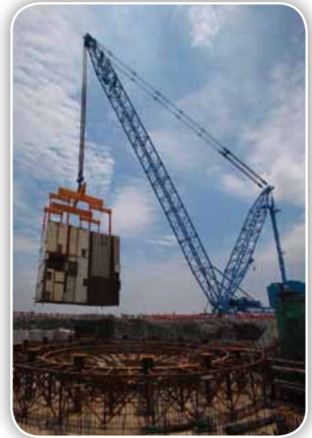
One of the world's largest cranes lifts the finished CA-20 module into place at the Sanmen AP1000 reactor site in China's Zhejiang province. (Photos: SNPTC)
