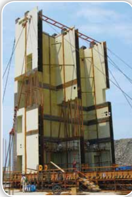
For very large modular structures, such as the CA-20 auxiliary building, submodules can be shipped to the site separately and assembled in an area close to the plant.
