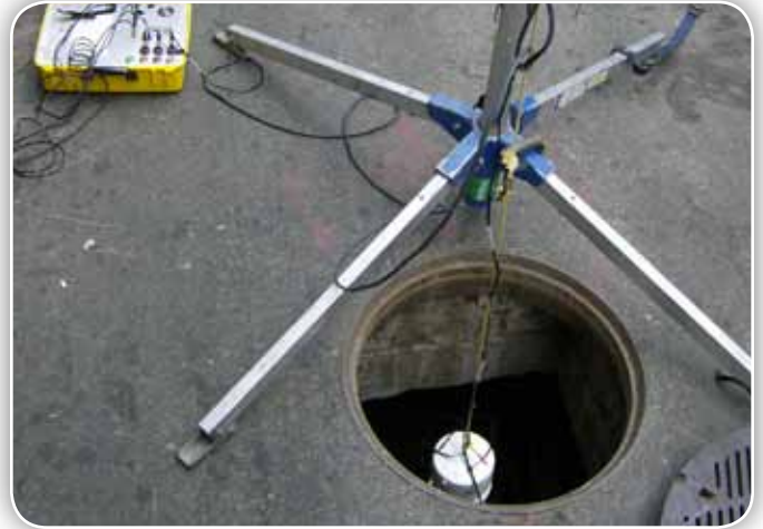
Lowered into a manhole, the detector's sensor pod can signal the presence of arcing before workers enter underground structures.
