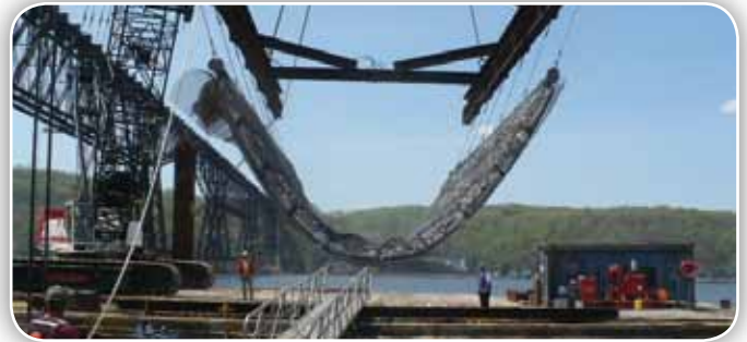
Sorbent-filled marine mattresses are lowered into the Hudson River to test their effectiveness in cleaning up coal tar residues.
