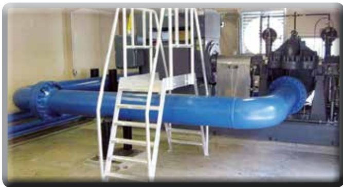
Main pump and motor assembly used at the jet pump facility. The pump has a capacity of 10,000 gallons per minute.
