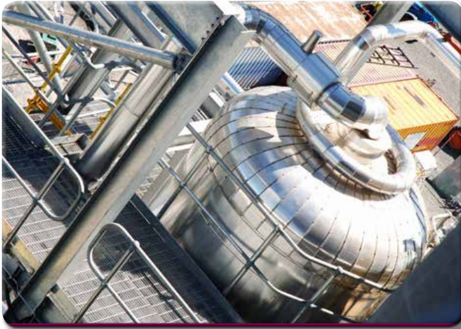
HRSG at the 400-MW Tallawarra KA26 combined-cycle power plant, Australia (Copyright: Alstom)
