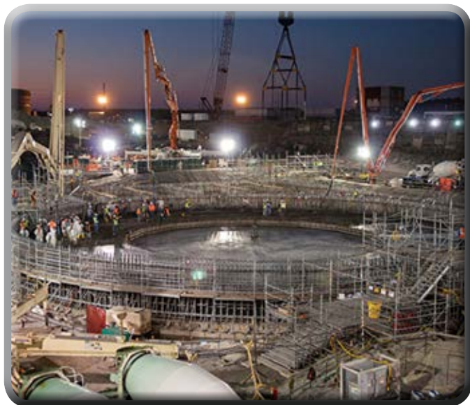
EPRI's field guide on concrete helped SCANA effectively monitor quality control procedures during concrete pad construction at the V. C. Summer plant. Photo courtesy of SCANA Corp.
