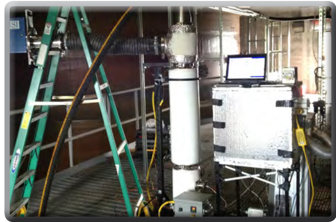
The quantitative aerosol generator (the white cylindrical device) delivers aerosol to an emissions monitoring system for calibration.
