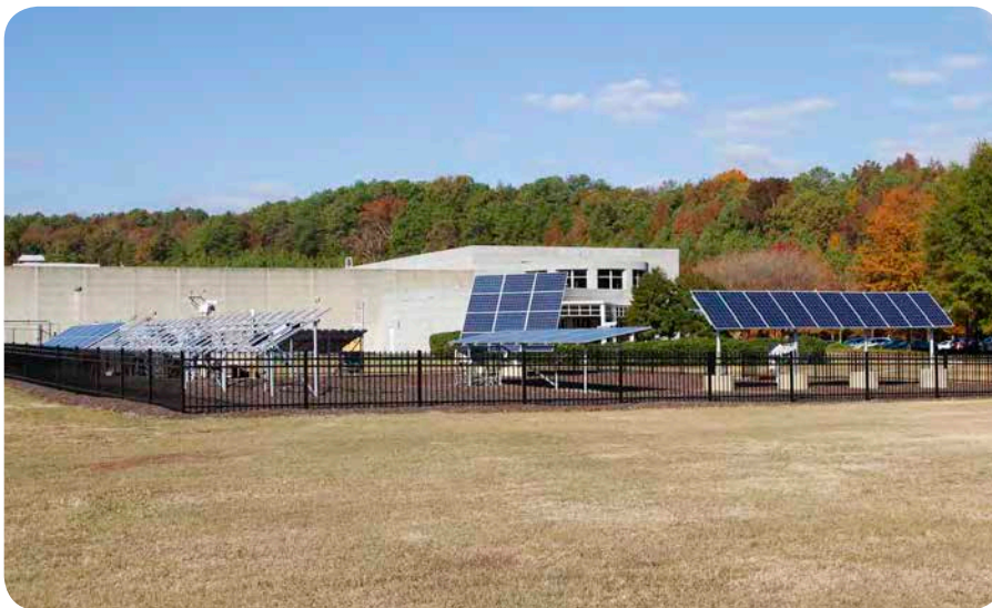
Solar arrays with different orientation and tracking methods at the research center
