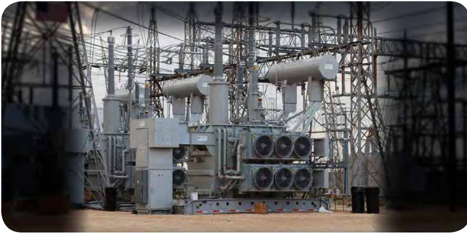
As part of an emergency drill with the U.S. Department of Homeland Security, EPRI, and others, the modular recovery transformer at this Texas substation was successfully deployed in just five days.
