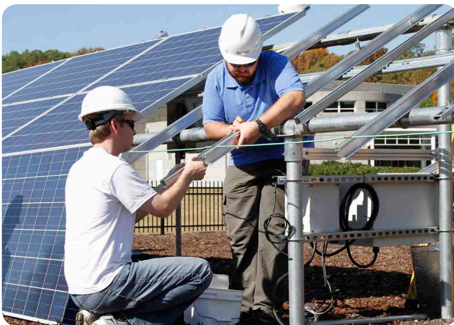
EPRI staff Chris Trueblood and Daniel Foster install components for the Center's soiling measurement station.
