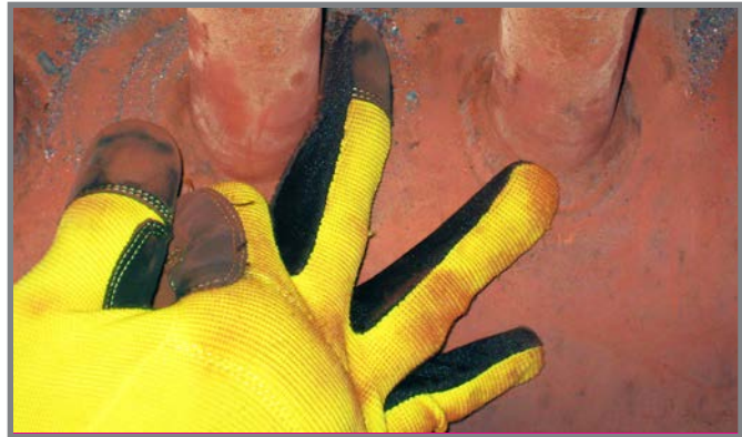
A glove equipped with the flexible eddy current array probe is used to inspect tube-to-header welds in a heat recovery steam generator.
