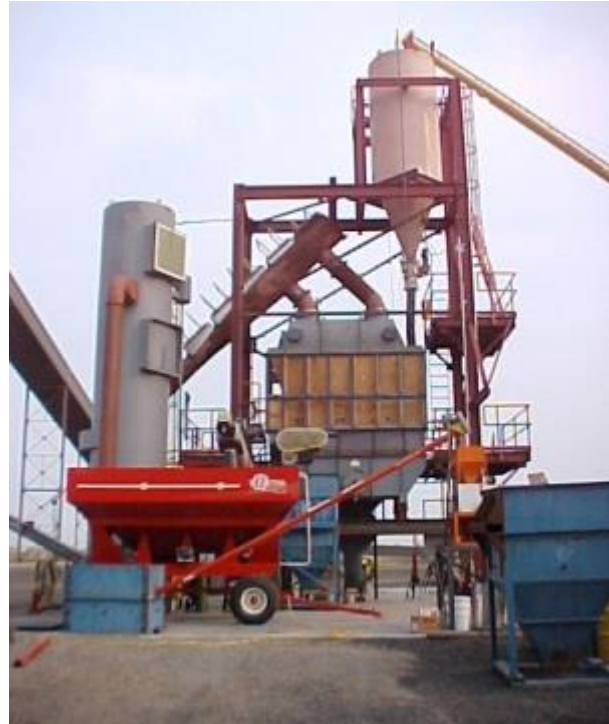
In 2003, six years before Great River Energy commercialized DryFining, this small-scale facility was built adjacent to Coal Creek Station.
