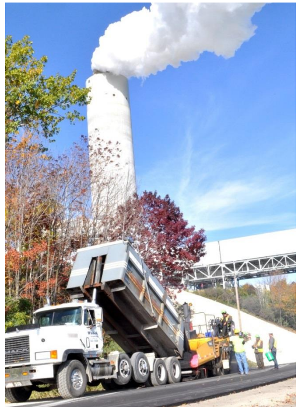
Proof of concept: After lab results pointed to the effectiveness of using fly ash as an ingredient in asphalt, We Energies field-tested ASHphalt by using it to pave a road at its Oak Creek coal plant.
