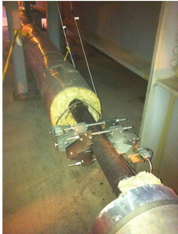
Components of the EPRI-Flexim flowmeter solution attached to a drain pipe in a heat recovery steam generator.
