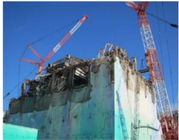
Clean-up of rubble at Fukushima Unit No. 3 in preparation for future fuel debris removal
