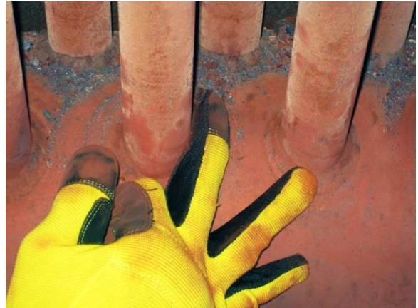
A glove equipped with the flexible eddy current array probe is used to inspect tube-to-header welds in a heat recovery steam generator.
