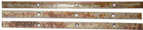
Corrosion on a set of strips that were not treated with film-forming products
