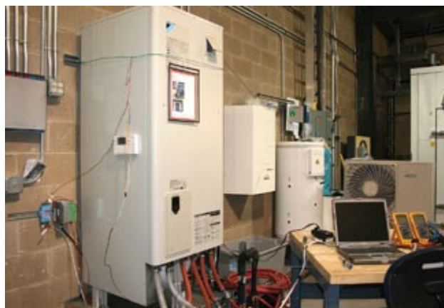
The Daikin Eco-Cute heat pump water heater, left, is instrumented for evaluation at EPRI's Living Laboratory in Knoxville, Tennessee. The high-efficiency unit also includes an outdoor component.
