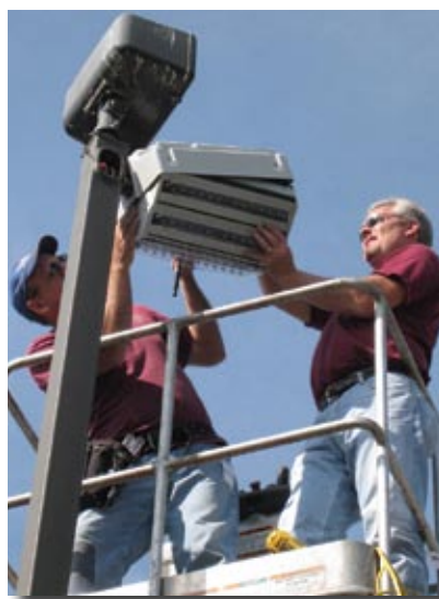
Engineers replace metal halide downlights with LED fixtures in the Living Laboratory's parking lot.
