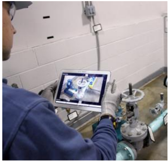
A plant technician uses the tablet technology to verify the completion of a valve alignment.
