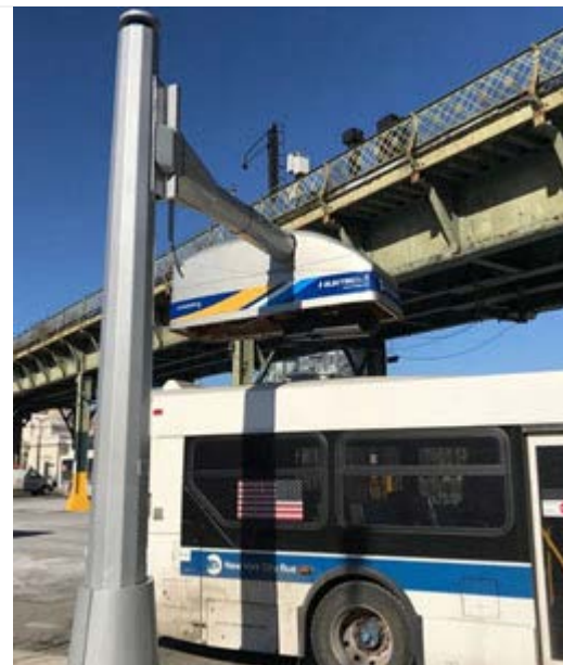
An overhead bus charger being monitored in the NYPA demonstration project.
