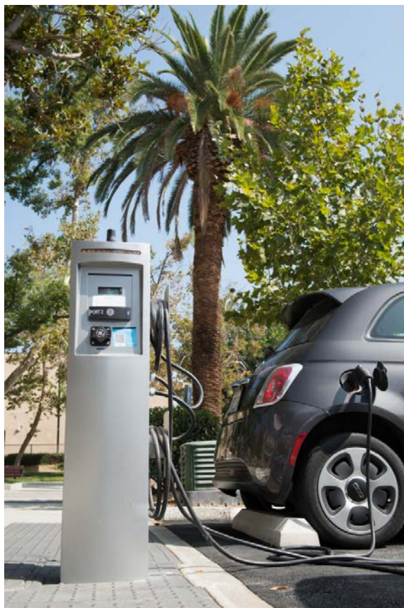
Southern California Edison installed this electric vehicle charger as part of its Charge Ready Program. Photo courtesy of Edison International.
