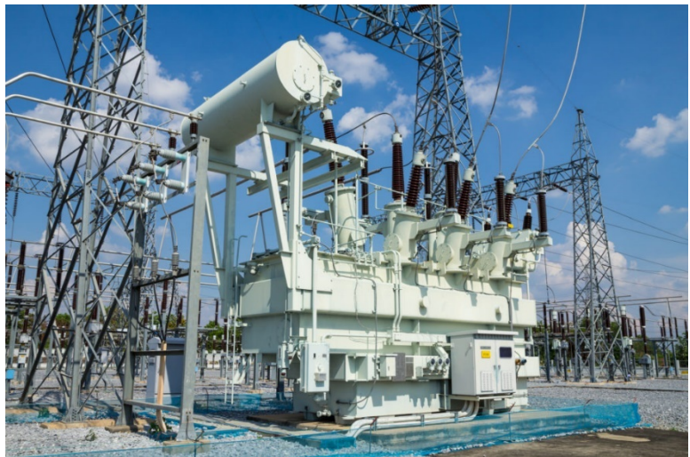
A bulk power transformer.
