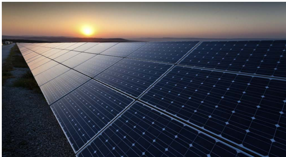
A large-scale solar power plant.
