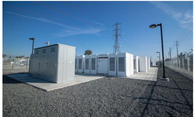
Southern California Edison’s Mira Loma Battery Storage Project can store up to 80 megawatt-hours of electricity. Photo courtesy of Ernesto Sanchez/Southern California Edison.
