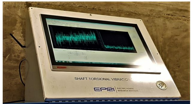
Readout from the monitoring system's interface at Bad Creek Hydroelectric Station.
