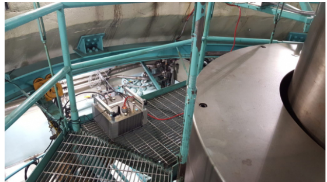
Stationary components of the monitoring system placed in the turbine room of Bad Creek Hydroelectric Station.
