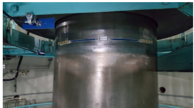
Monitoring components deployed on the turbine shaft at Bad Creek Hydroelectric Station.
