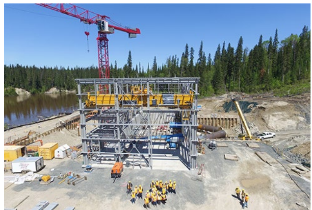
Construction of the Peter Sutherland Sr. Generating Station, a hydropower facility completed in 2017. Photo courtesy of OPG.
