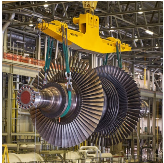
A turbine being hoisted as part of the refurbishment of Darlington Nuclear Generating Station. Photo courtesy of OPG.
