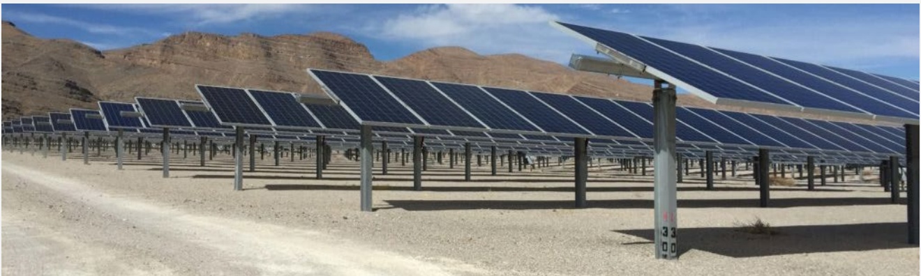
Researchers conducted electroluminescence imaging on PV modules at this commercial PV plant to better understand the link between module defects and power degradation.
