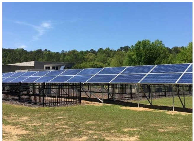
The PV modules in this array at the Southeastern Solar Research Center were subjected to accelerated aging tests before being installed outdoors. Photo courtesy of Southern Research.
